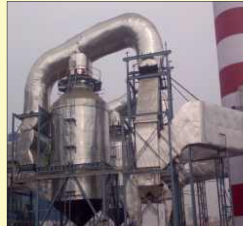
Nye Tray Wet Scrubber with RCC Clarifier and Mechanized Slurry Handling at one Sugar unit
