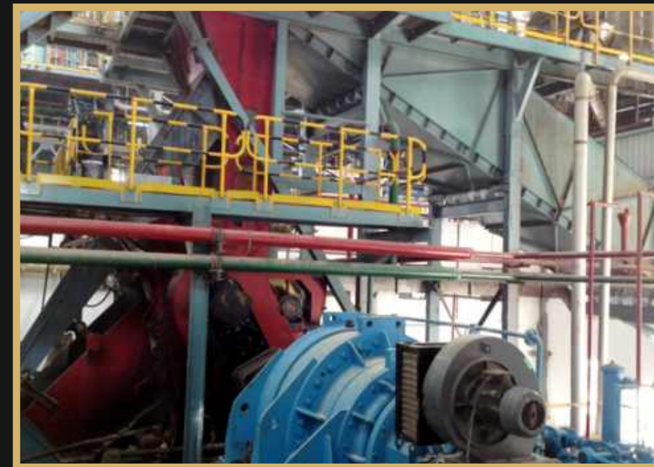
40''X80'' Two Roller Enmill Extraction Mill Installed at IJT-HPCL Biofuels Ltd., Sugauli & Lauriya (Bihar)
